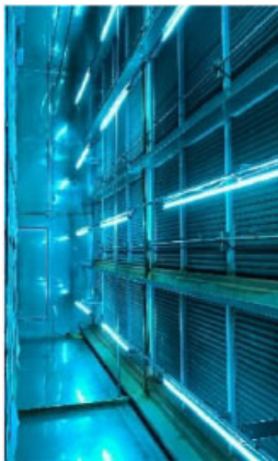
Air Handler Disinfection
